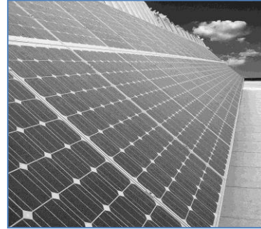
Photovoltaic plant, Hangar 7
